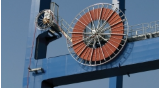
A Pull & Store reel application at Copenhagen Port, Denmark
