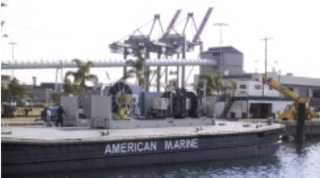
Cavotec reel mounted on a maritime power supply application
