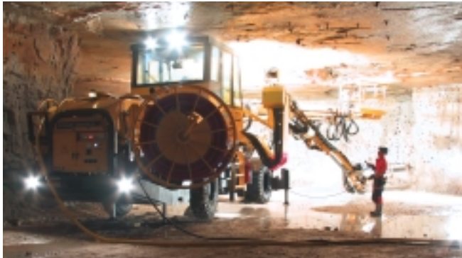
Cavotec reel at work in a Swedish mine
